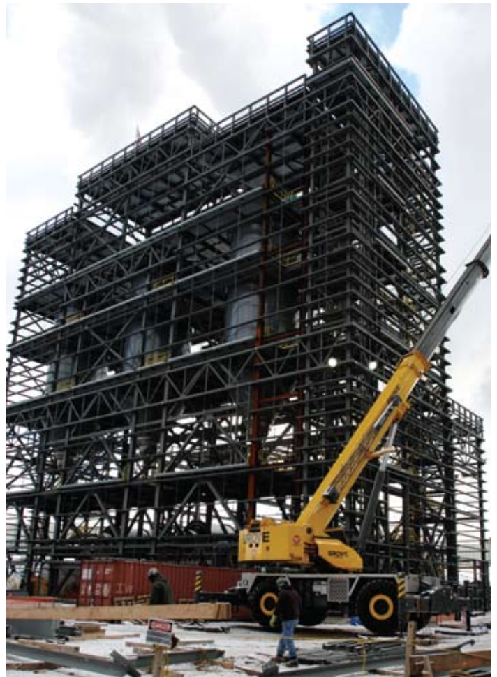
Flue gas desulfurization equipment, commonly known as scrubbers, controls 95 percent of the sulfur dioxide emissions at our power plants.
