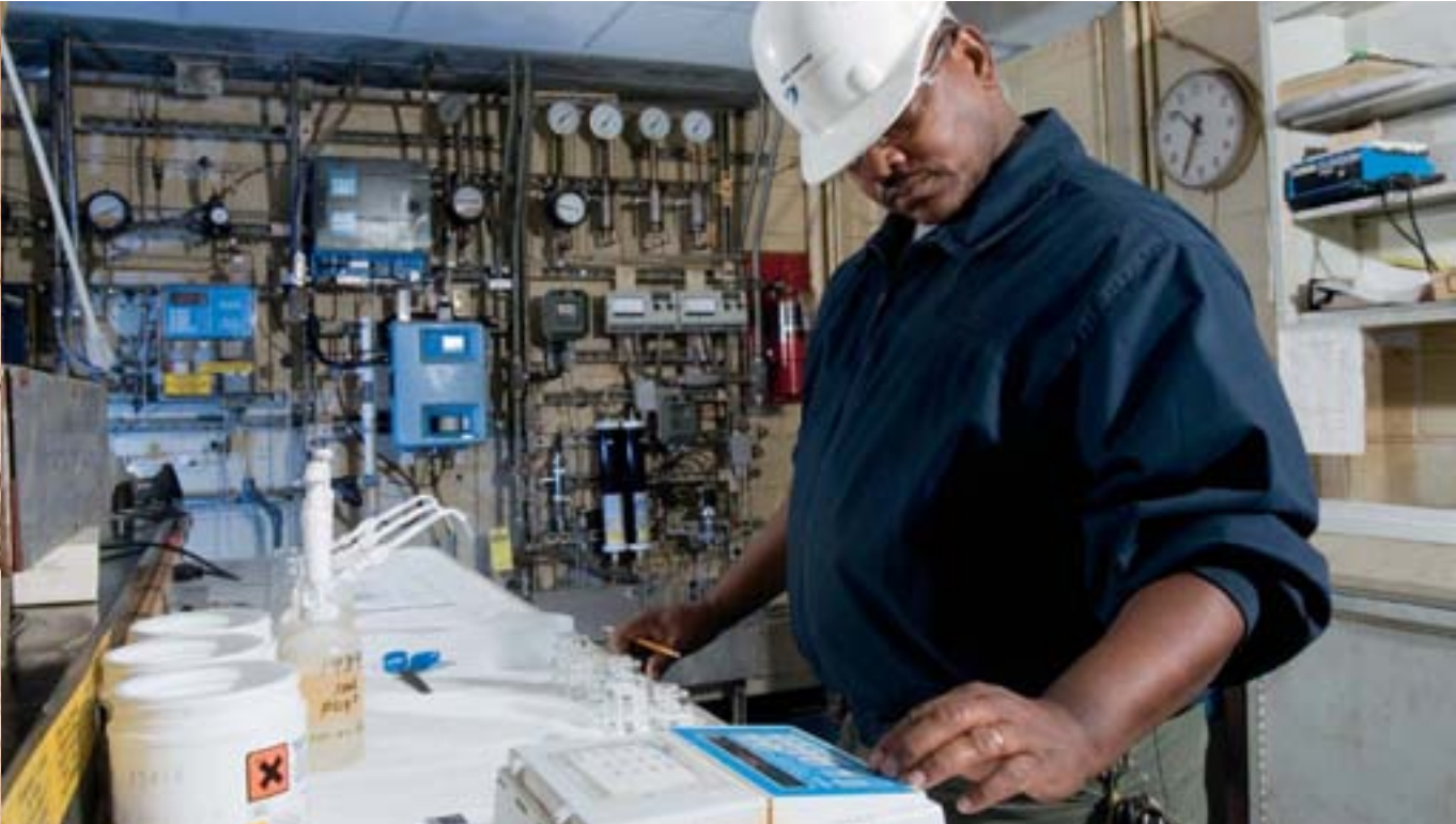
Operator Ben Stallworth works at our on-site energy facility that powers the Kimberly-Clark tissue mill in Mobile, Ala.
