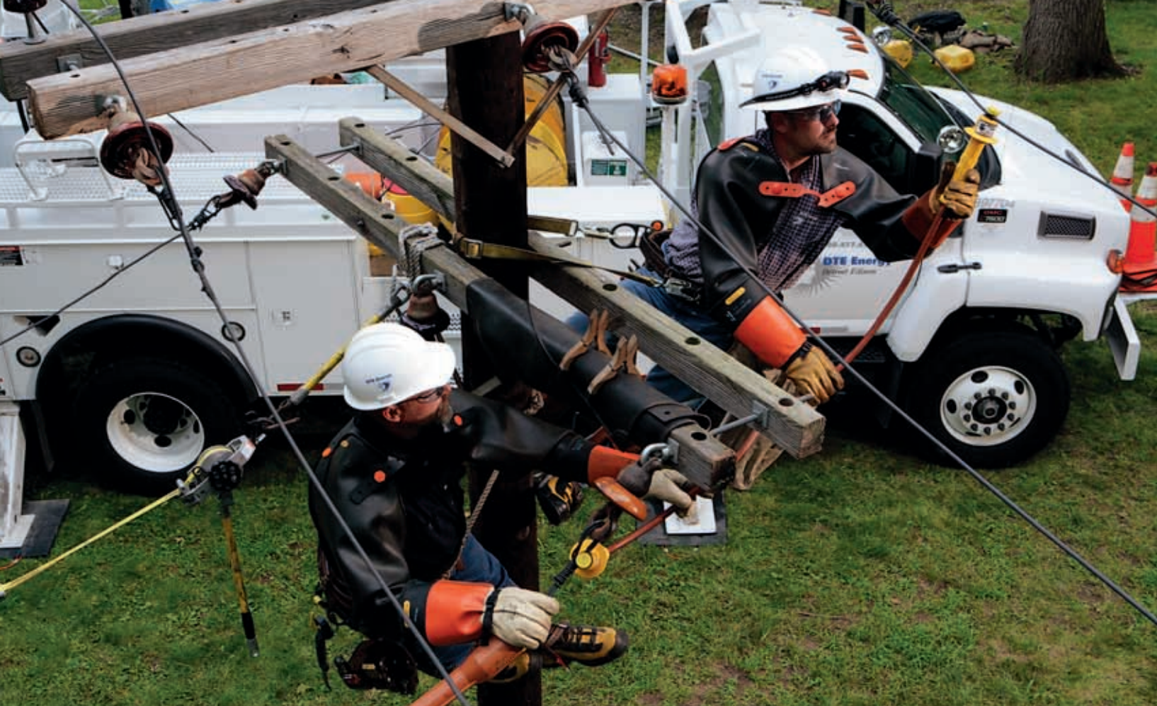
Linemen Charles Dortenzio and James Shaw work on a distribution circuit. This work requires trimming 1,200 trees, repairing 101 pole tops and replacing roughly eight outdated poles.
