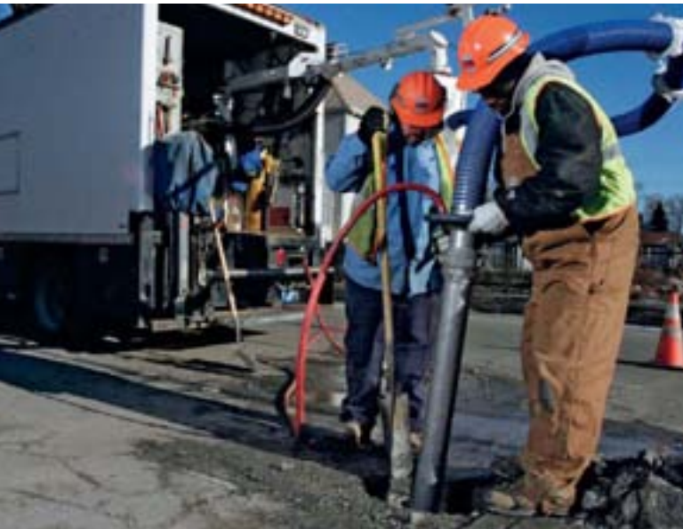
DTE Energy is a leader in keyhole technology designed to minimize gas leak repair time and costs. Fitters Fred Drys (left) and Alphonso Hill.
