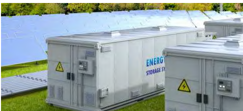
SLOCUM BATTERY ENERGY STORAGE
