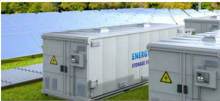
SLOCUM BATTERY ENERGY STORAGE
