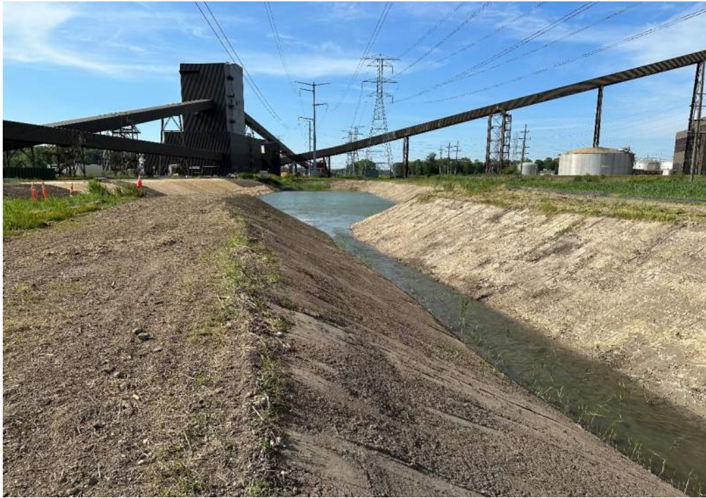
Photo 14: W side of N channel, CCR removal & overexcavation complete, topsoil applied to E side, looking S (7/11/2023)
