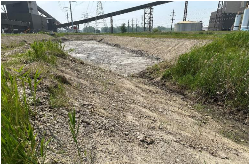
Photo 13: E side of N channel, CCR removal and overexcavation complete, looking S (6/29/2023)
