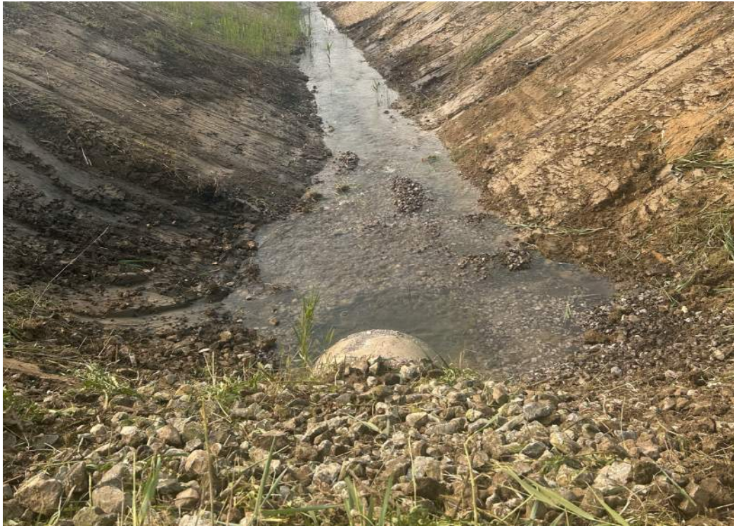
Photo 18: North end of N. channel, remaining CCR removal and overexcavation complete, looking S. (7/19/2023)
