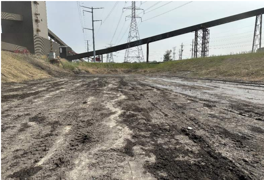
Photo 7: Top of hardened CCR layer in Diversion Basin bottom (6/6/2023)
