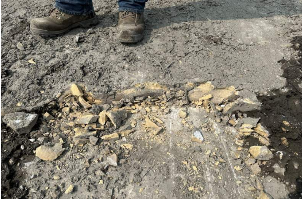
Photo 6: Hardened CCR material discovered below initial CCR removal (6/6/2023)
