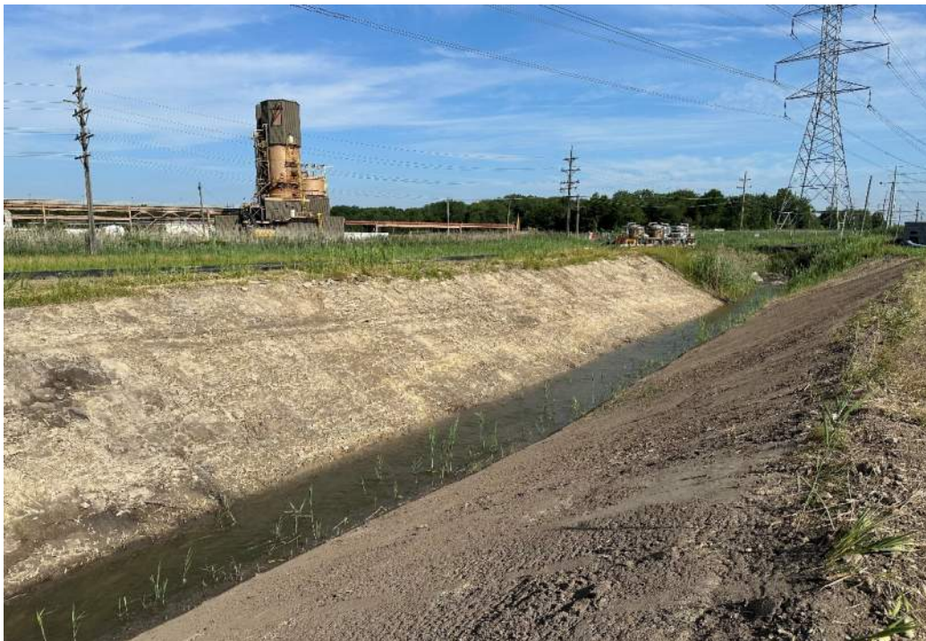
Photo 15: W side of N channel, CCR removal & overexcavation complete, topsoil applied to E side, looking N (7/11/2023)
