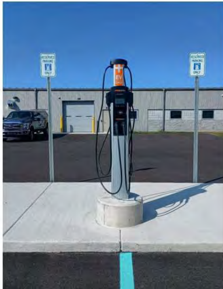
Two Public Level 2 EV chargers for Walled Lake School
