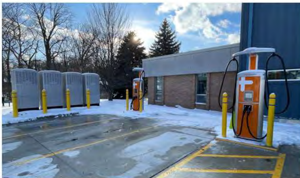
A DC fast charging installation supports rapid turnaround for University of Michigan Ann Arbor fleet vehicles, enabling multiple high-power sessions throughout the day while optimizing site energy use.
