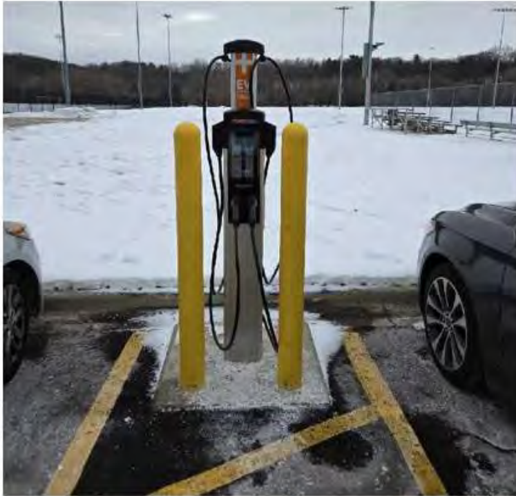
A Level 2 fleet charging installation supports daily operations for University of Michigan Ann Arbor vehicles, enabling reliable overnight charging and efficient energy use.
