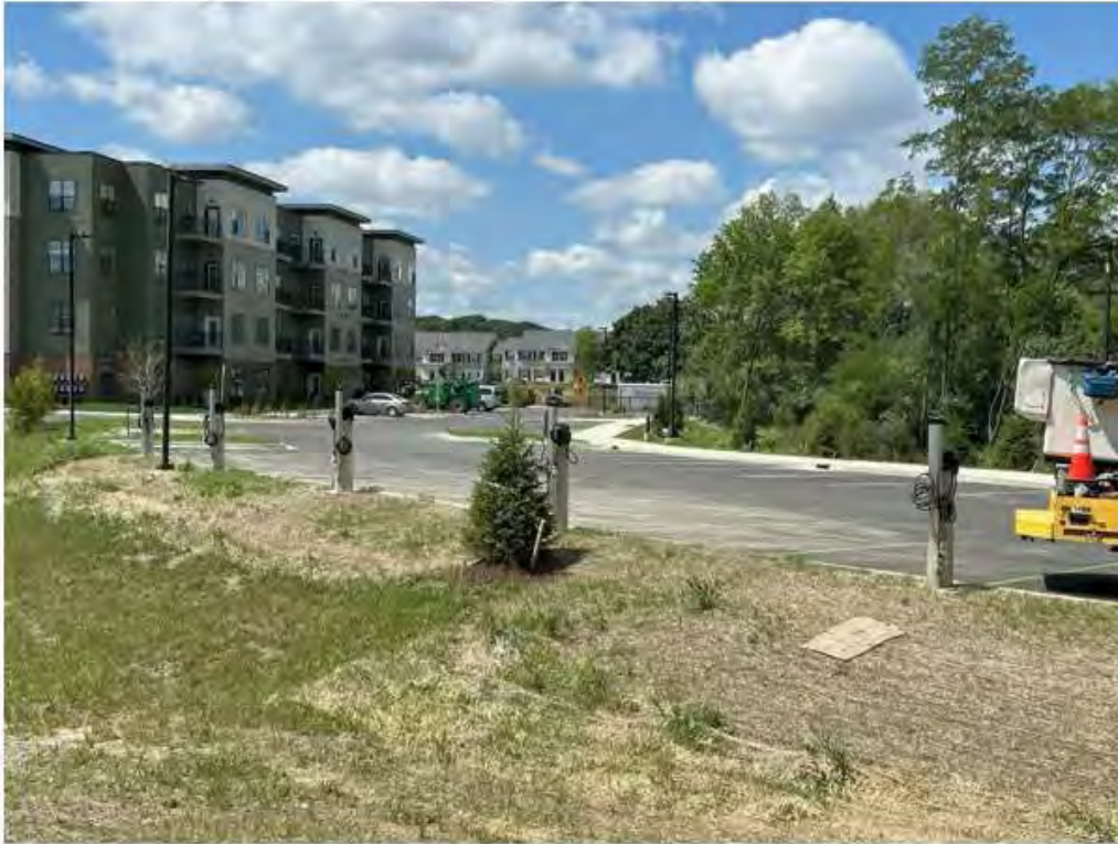
Ten Level 2 EV chargers for a new development Low-Income property with 295 units
